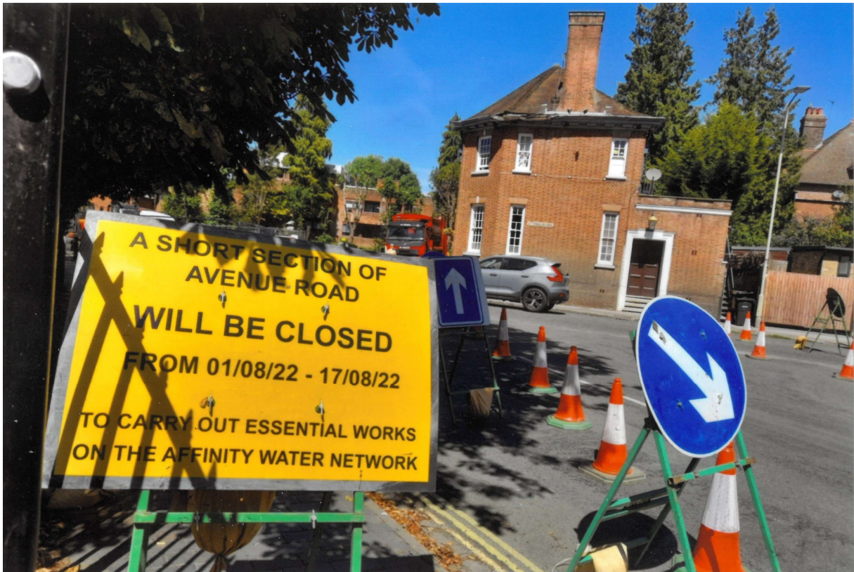
New water pipes at The Cricketers, junction of Stonecross, Harpenden Road, Avenue Road, St Peter's Street, Summer 2022
